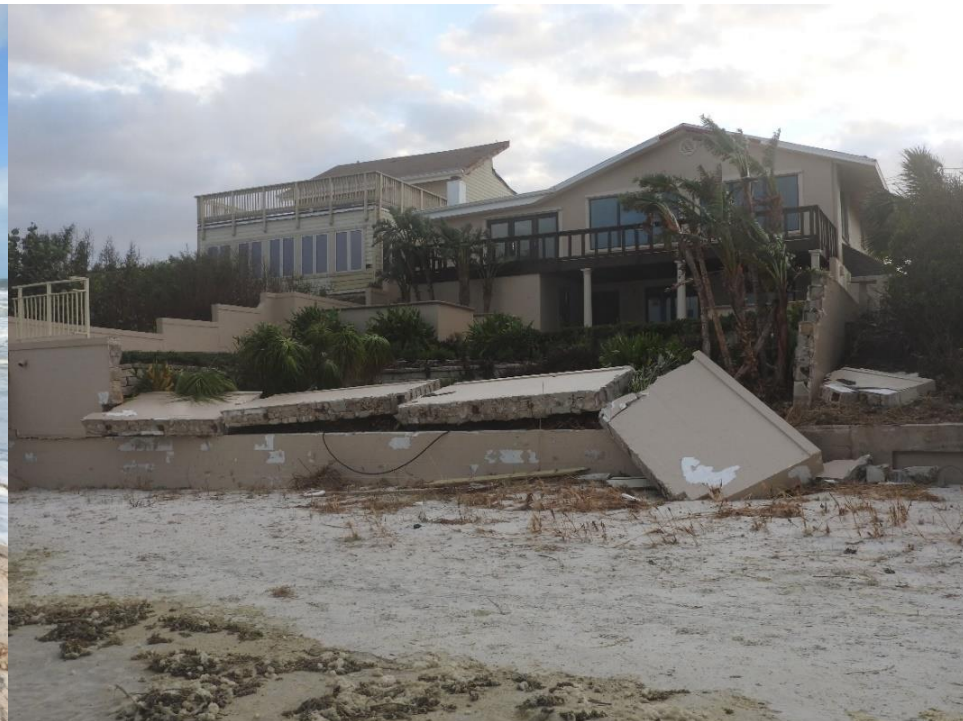
Wilbur-by-the-Sea Wall Damage
