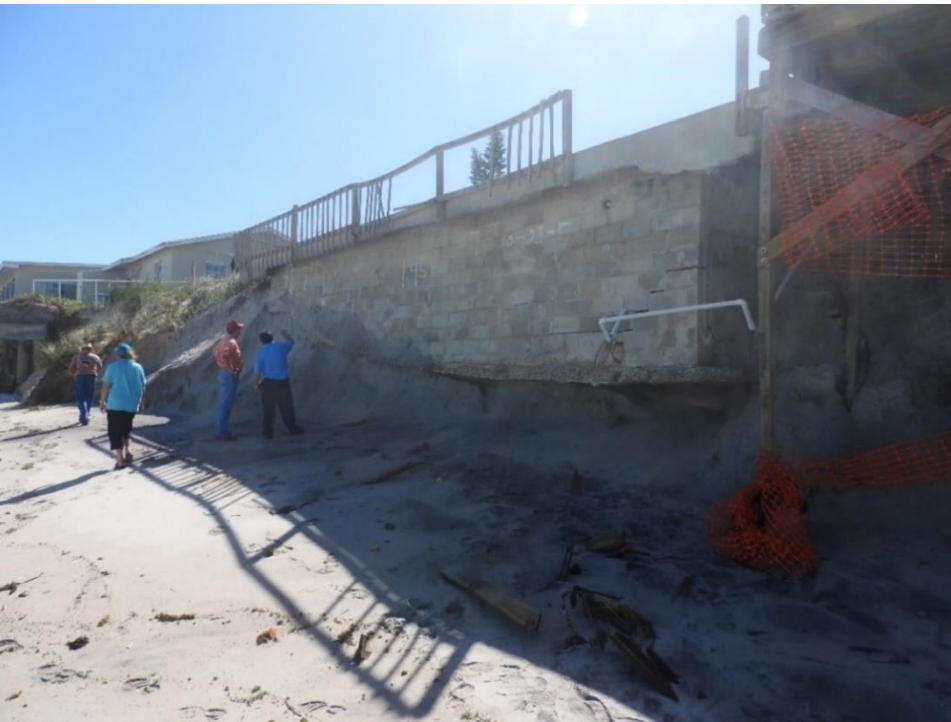
Swimming Pool Undermined
