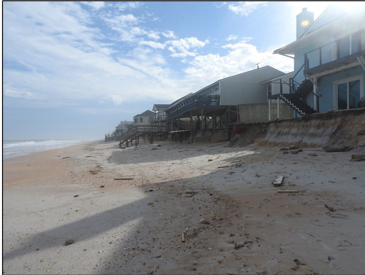
Major beach and dune erosion in South Ponte Vedra Beach, erosion condition IV, near R-86
