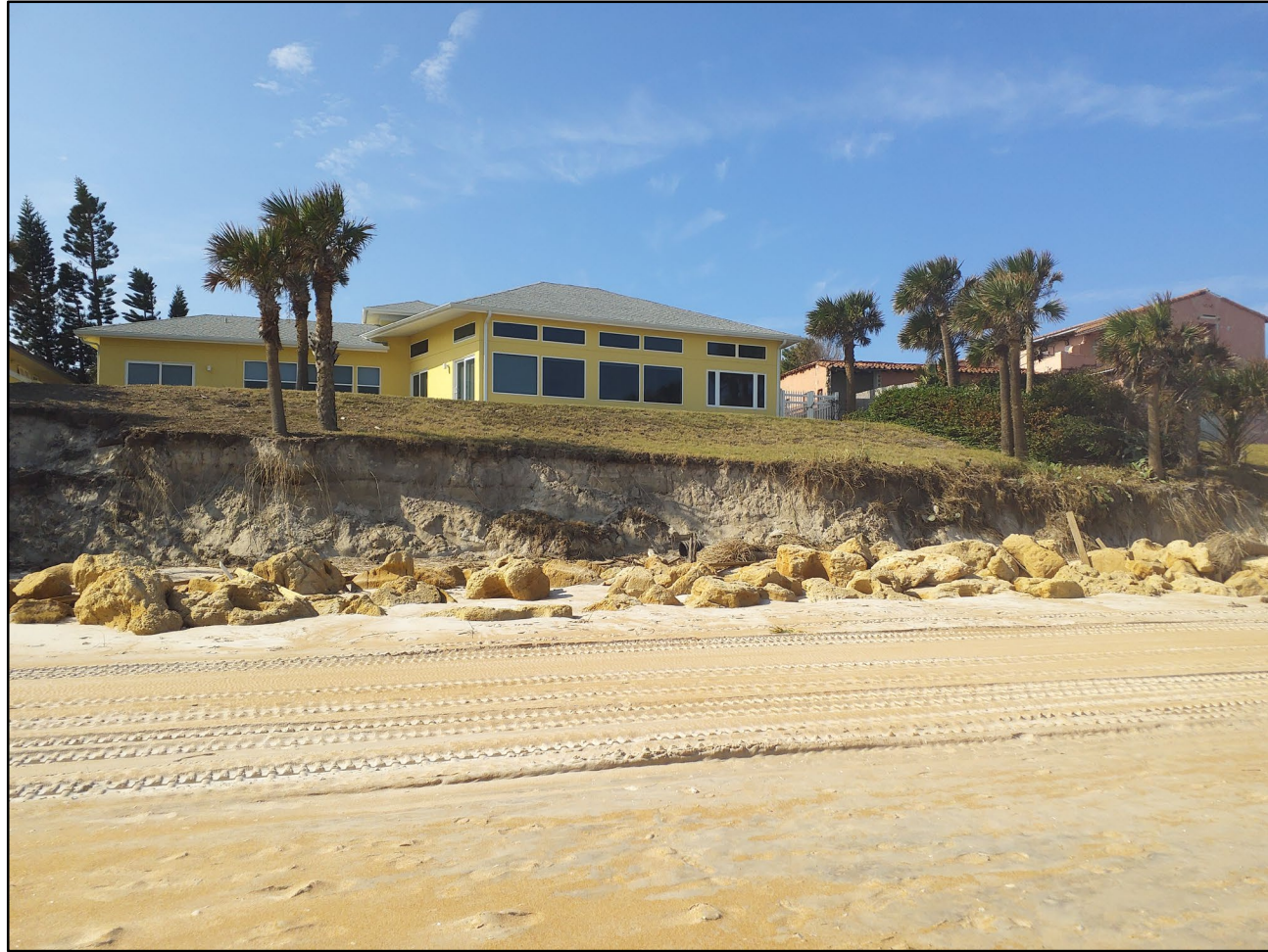
Major beach and dune erosion at Ormond Beach, erosion condition IV, near R-55
