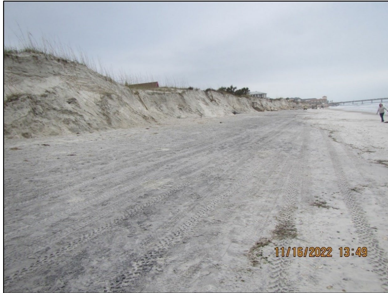
Major beach and dune erosion at St. Augustine Beach, erosion condition IV, near R-144
