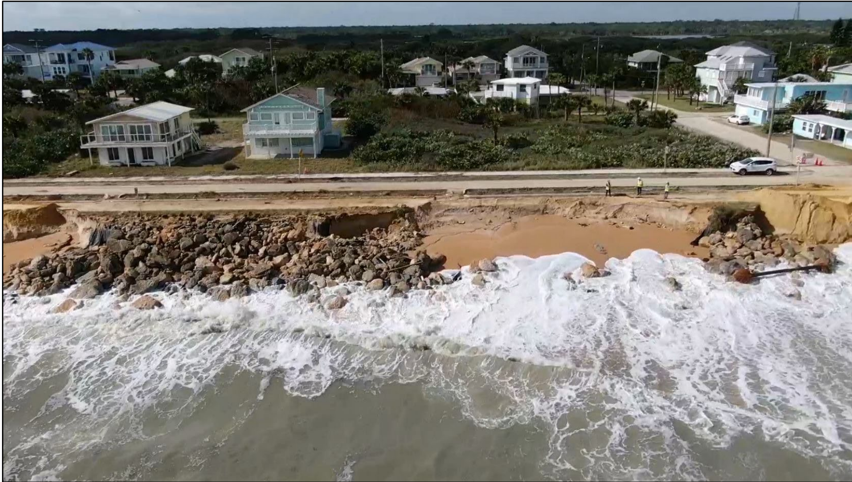
Hurricane Nicole's beach and dune damages (condition IV) to A1A in Flagler Beach (R-88, 17 th St. South), photo by Civil Air Patrol
