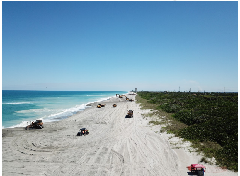
Construction of the Patrick Space Force Base segment was completed by The Dutra Group in April of 2021. Credit: U.S. Army Corps of Engineers
