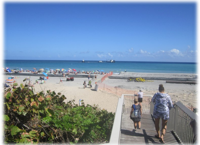
February 2, 2014, at Ocean Ridge in Palm Beach County. Happy beach users on the new beach (left, center) and the Dredge Savannah (Marinex) in the background working to complete the project. Progress of work is from left to right.
