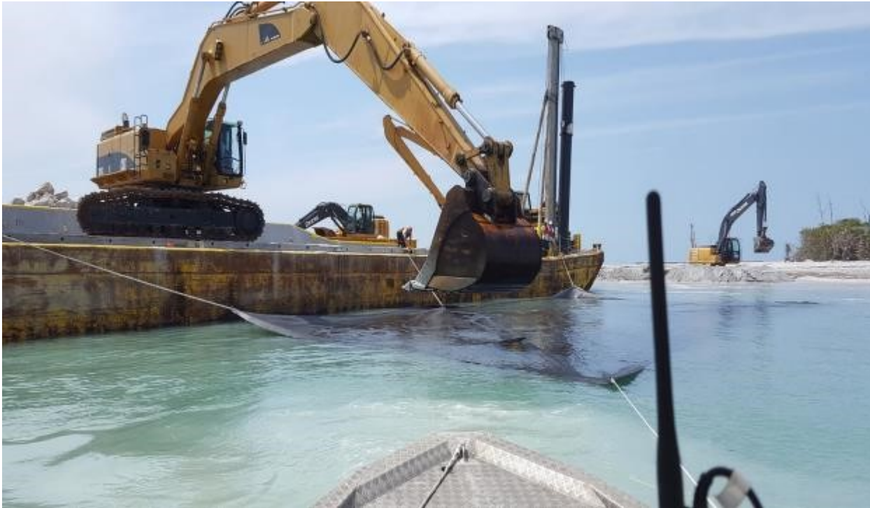
Figure 11. 2017 Project: Installing Geotextile Fabric and Placing Bedding Stone to Sink into Place as Foundation of Groin.
