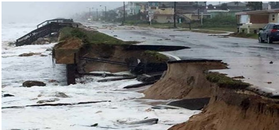
Figure 2: Damage to SR-A1A after Hurricane Matthew in 2016.
