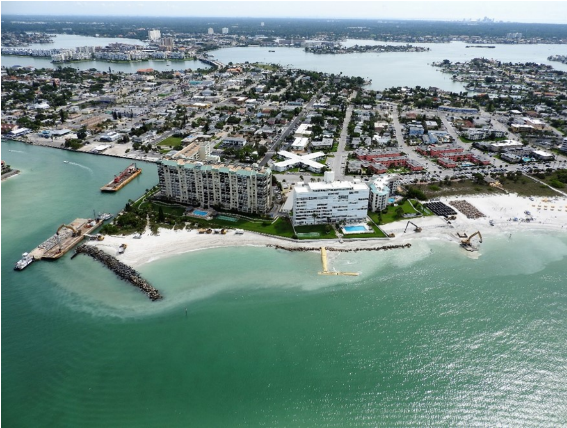
Figure 3. Construction of the rock groins at Upham Beach – Pinellas County in May 2018 adjacent to Blind Pass, between R144 and R145. Photo by Guy Weeks.
