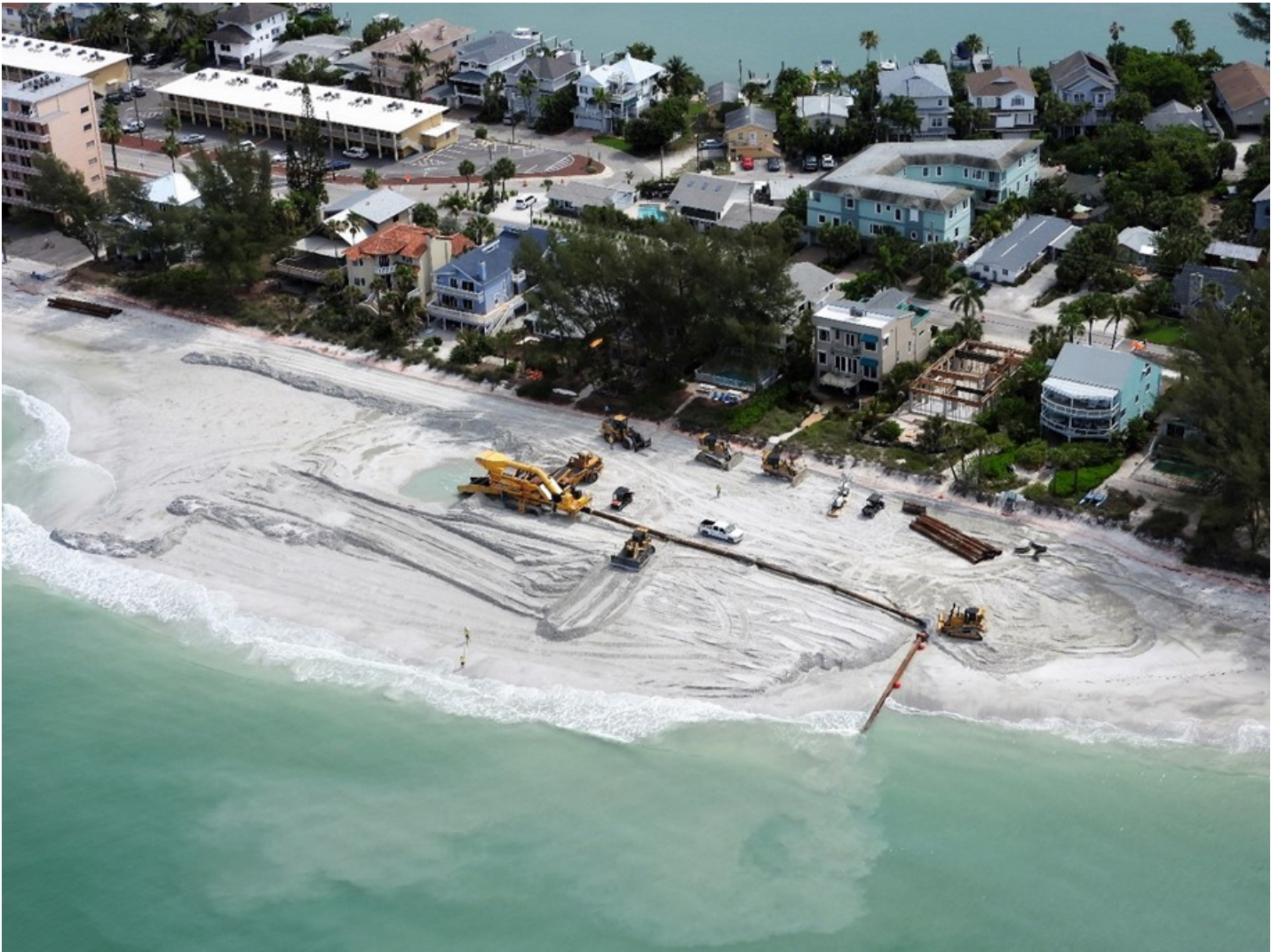
Figure 2. Construction of the Pinellas County Shore Protection Project on Treasure Island in May 2018, near R139.5. Photo by Guy Weeks.
