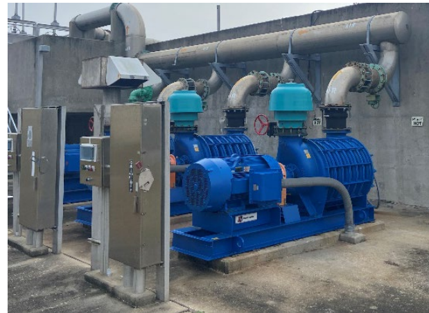
Blowers, Motors and Control Panels
