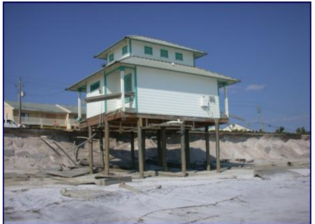
Miramar Beach Regional Beach Access restroom following Hurricane Ivan
