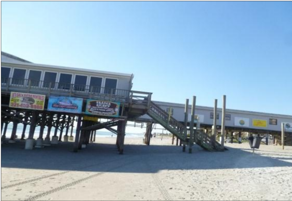
Brevard County, North Reach, Meade Ave. (Cocoa Beach Pier), October 31, 2012. Beach loss measured vertically on the pier pilings as much as two feet.
