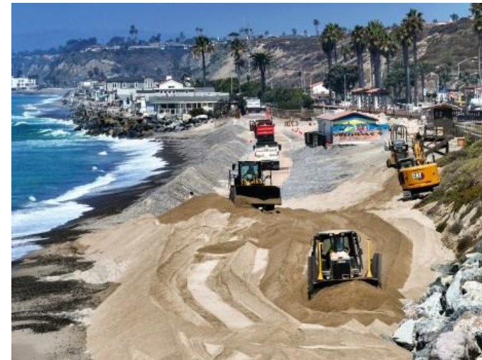
Beach nourishment of North Beach in San Clemente, August 2024 Source: The Orange County Register
